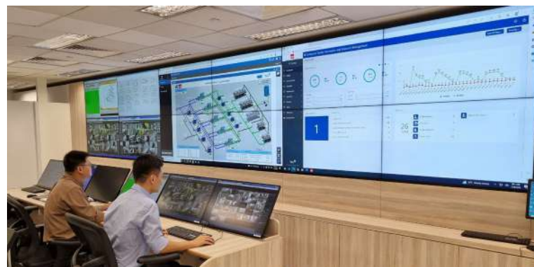
Integrated Building Management System Dashboard
